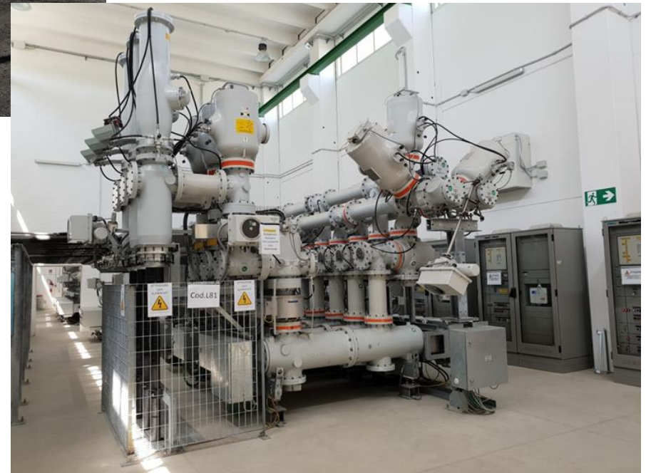
Gas Insulating System
