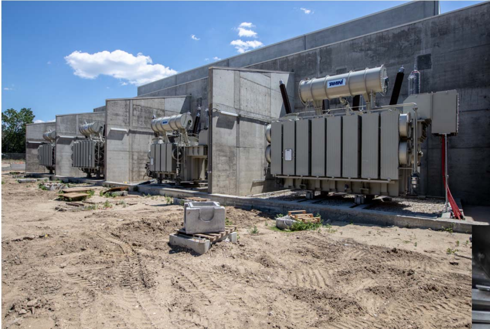
4+4 external oil transformers
